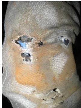
Fig. 2.2.3 (b) Damage on the cable protective sleeve
